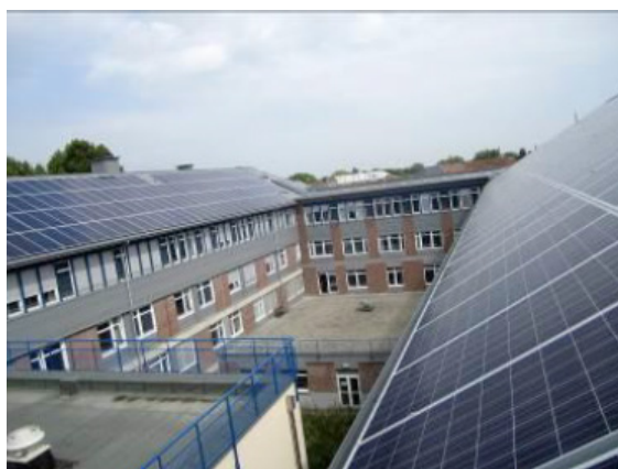
Illustration 18: Photovoltaic system connected to the 425kW grid in Soignies, Belgium, in an existing hospital, which reduces electricity costs by 95% Source: TECSOL 2014
