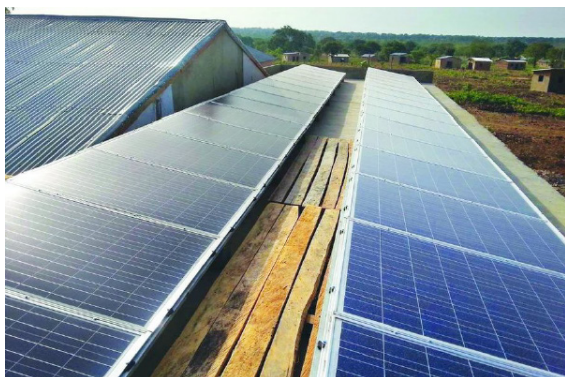
Illustration 17: Hospital that received a donation of a 19kW off-grid system in northern Benin, which supplies the warehouse and the local cafeteria Source: MORAGUES, 2015
