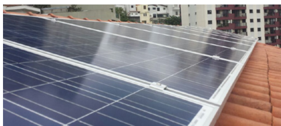
Illustration 20: Photovoltaic system connected to the grid with 2.34 kWp of panels and 3 kW inverter, located in São Paulo, Brazil, at the headquarters of the Hospital Research Institute Jarbas Karman Source: Solstício Energia, 2016
